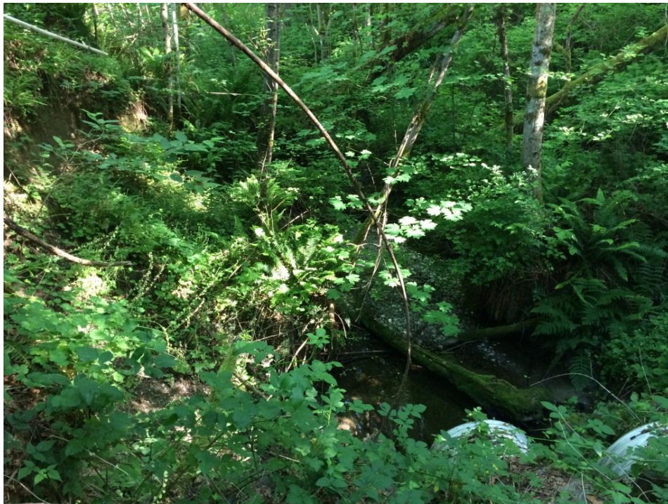
Photo 2: Facing southeast along stream within vegetated ravine (approx. 100-ft downstream of site). Outfall of twin culverts in bottom right of photo. Visible evidence of ravine erosion within 20-30 ft of stream, in upper left of photo.
