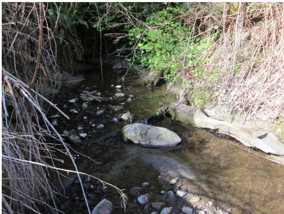
Photo3: Facing west along stream from inlet of box culvert which passes beneath 18 th Ave NE.
